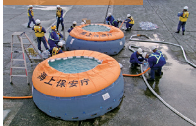
Water supply support
